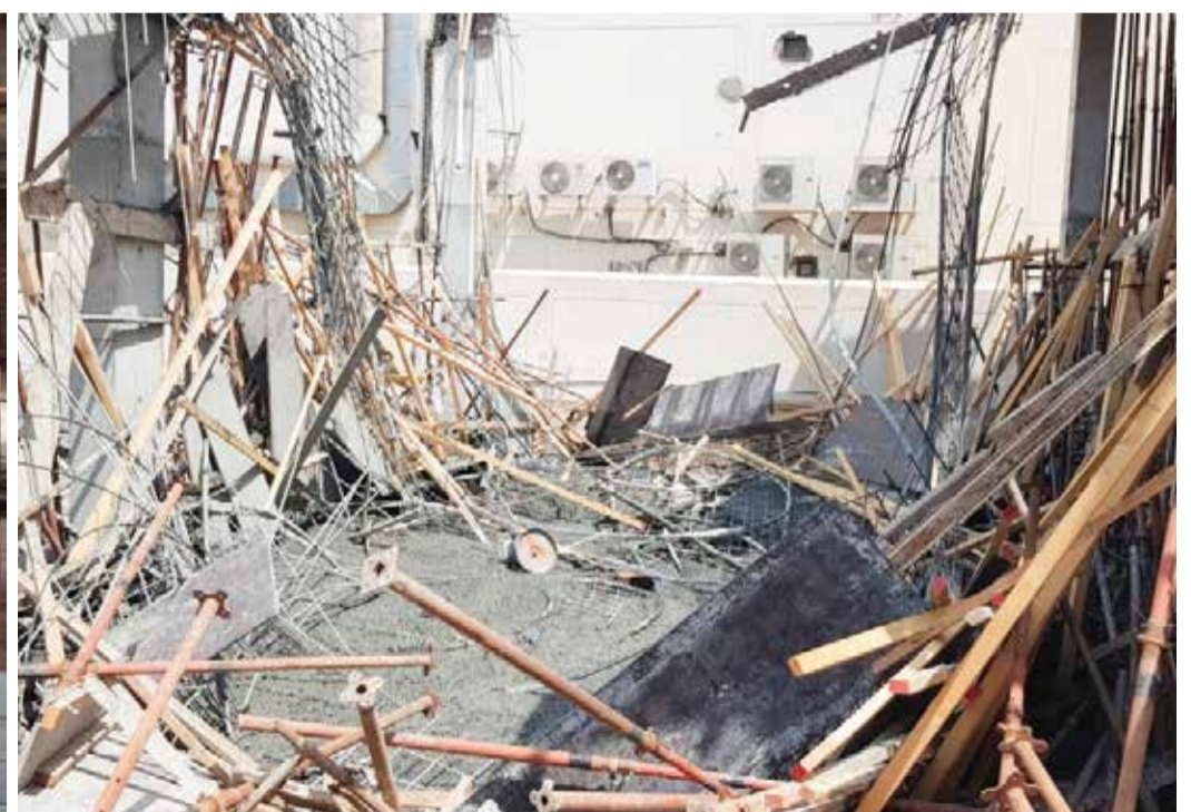
The remnants of the structure that collapsed.
